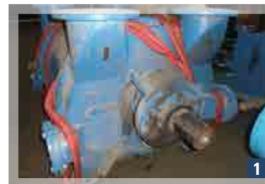
1 Pompa da revisionare tipo Cutes CE1. Vacuum pump to repair type Cutes CE1.
