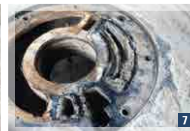
7 Testata intasata. Clogged end shield.
