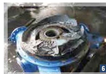
6 Disco distributore e testata intasati. Clogged port plate and end shield.
