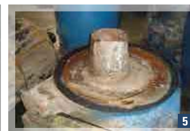
5 Coni distributori incrostati. Encrusted port plates.
