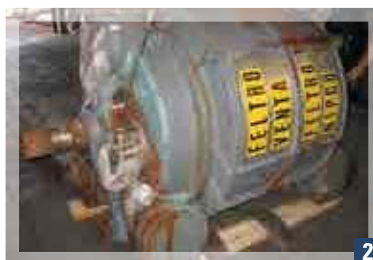
2 Pompa da revisionare. Vacuum pump to repair.
